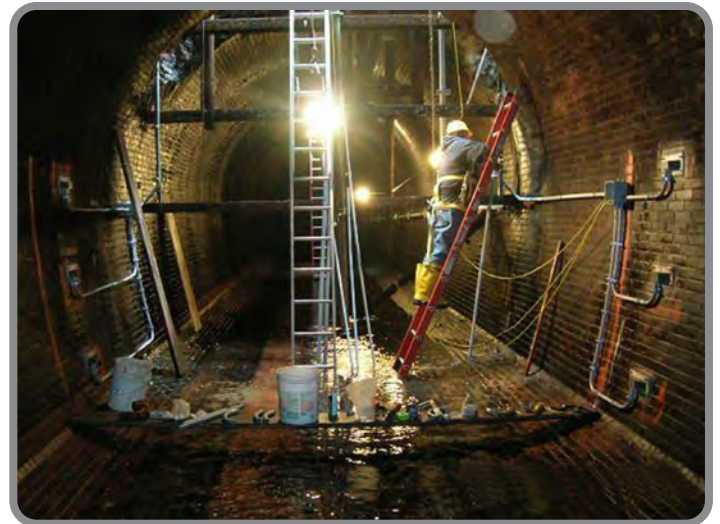
Installation in 12' diameter aqueduct (10 - 290MGD), Dunwoodie Project, Yonkers, N.Y. Three chordal transit-time paths with ultrasonic level sensor
